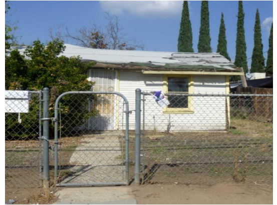
Example of Arvin Housing in Dilapidated Condition
