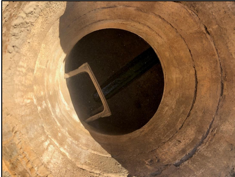
Figure 6.9 – Example of Manhole Recommended for Repair
