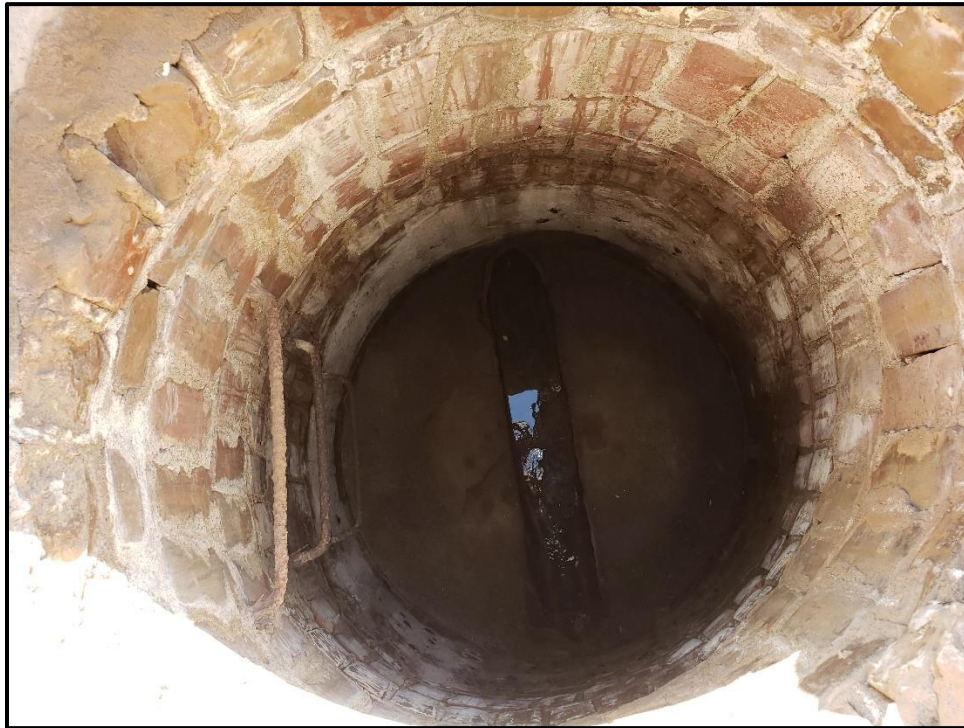
Figure 6.12 – Example of Manhole Recommended for Replacement
