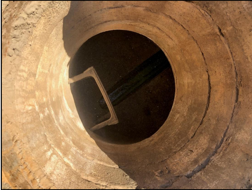
Figure 6.13 – Example of Manhole Recommended for Repair
