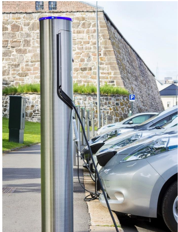
Figure 1. A line of easily visible Level 2 EVCS charging vehicles next to a pedestrian path.
