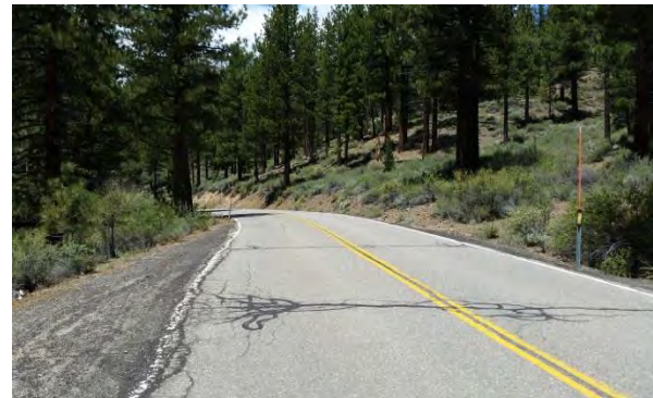
Photo 10. Example of Hot Springs Road pavement deterioration, facing west.
