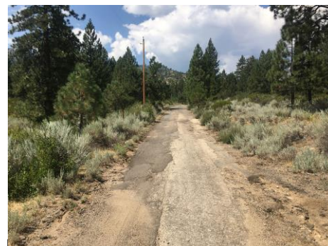
Trees/vegetation near driveways can impede egress
