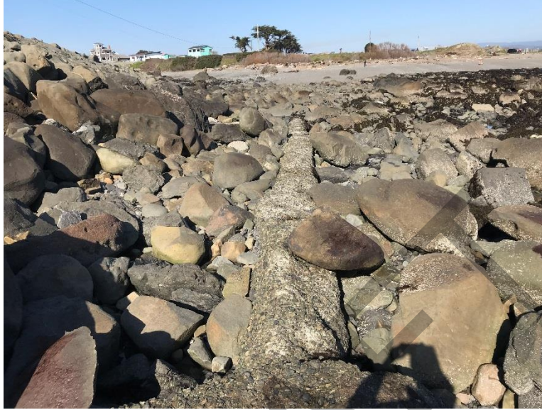
Feature 2, Concrete cover over 18/12-inch outfall. Concrete cover is in good condition.
