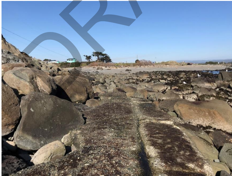
Feature 2, Concrete cover over 18/12-inch outfall. Concrete cover is in good condition.
